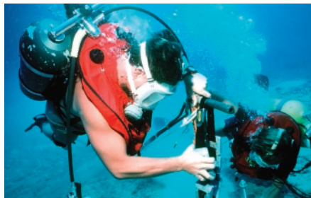
Remote video captured by cameras mounted to subsea divers' helmets provides pipeline managers a first-person perspective of the problem
